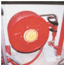
Fig. 5: Fire hydrant/hose reel
