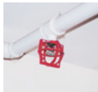
Fig. 6: Automatic sprinkler system
