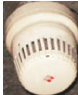
Fig. 4: Fire/smoke detection system
