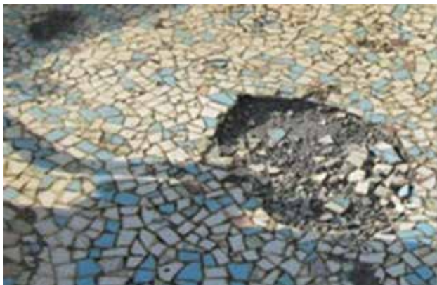
Fig. 7: Cracks developed in China mosaic waterproofing system
