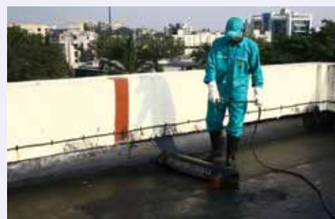
c. Torching the membrane by acetylene gas and pressing hard on the surface
