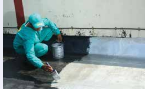
h. Finishing with aluminium coat for non-foot traffic or else screeding for foot traffic
