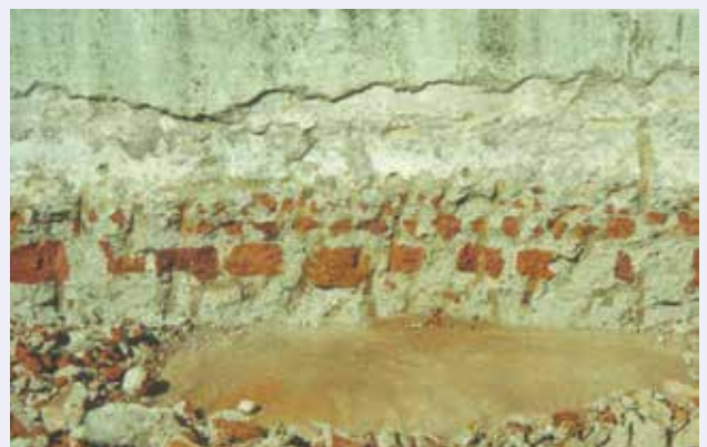
Fig. 6: Three layers of Brick-bat-coba increasing the dead load on the structure
