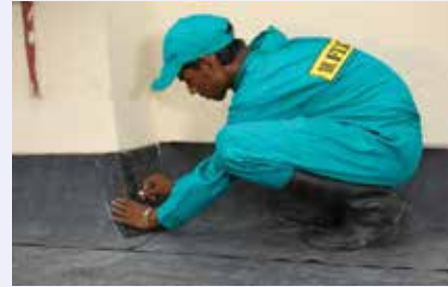
Fig. 16k: Marking on the membrane for splicing of cut piece at the corner junction
