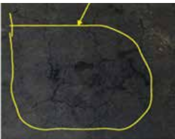
Fig. 12: Cracks in existing floor
