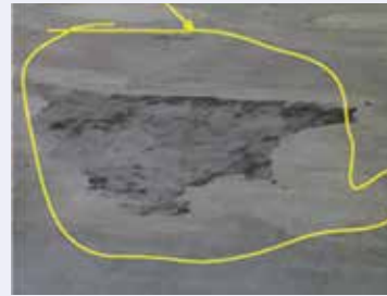
Fig. 13: Debonding of floor surfaces due to wear and tear
