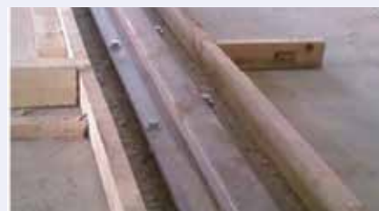
Fig. 2: View of form work and the rail being placed firmly before grouting
