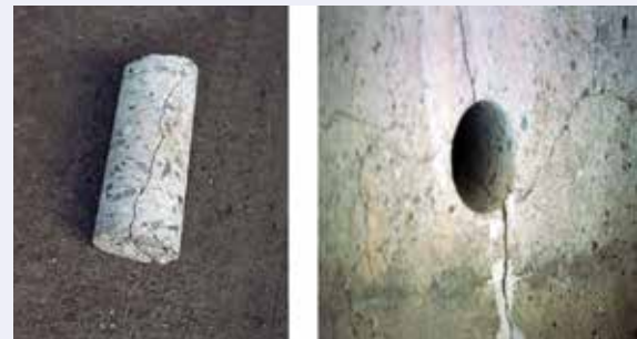
Fig. 7: Core sample taken from crack area
