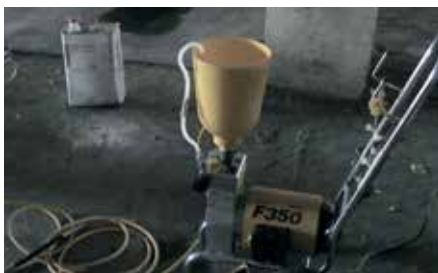
Fig. 2 b: High pressure Injection pump
